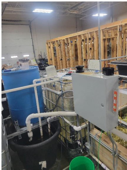
Electrical components of the aquaponics system
